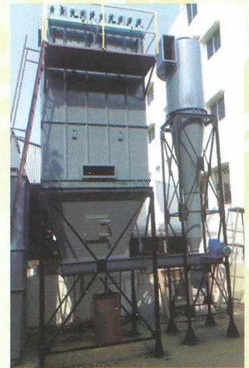
BAG FILTER WITH CYCLONE DUST COLLECTOR SYSTEM
